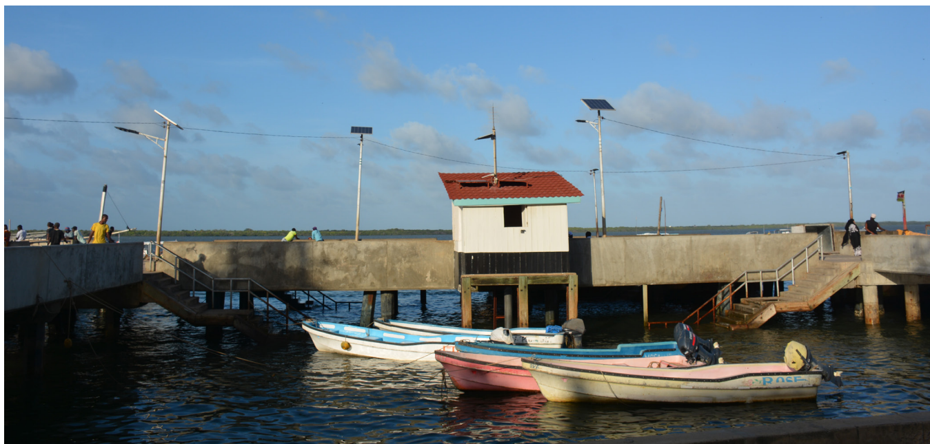
Solar panels at the Lamu Jetty in Lamu Old Town © SEI
